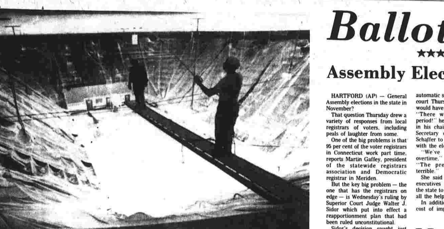
Hitting the High Spots. Painters use a platform supported by cables some 60 to 70 feet above the pool at Yale's Payne Whitney Gymnasium to paint the ceiling as covering protects seats. (AP photo)
